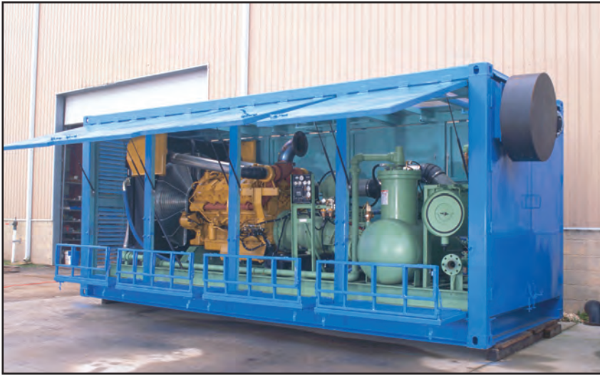
■ Containerized diesel-driven feed air compressor.
