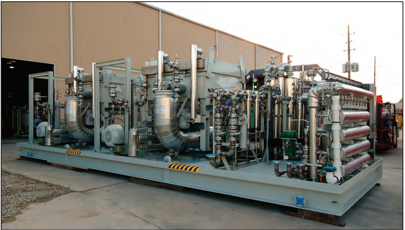
■ Hi-spec offshore instrument air and nitrogen plant with dual feed compressors.
